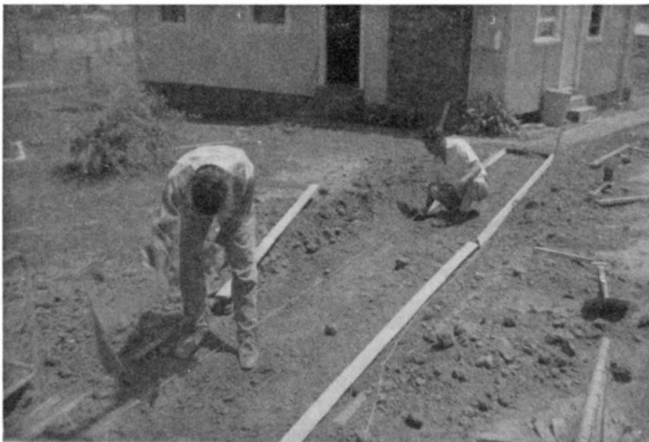
Dan Kelly and Willie Davis on formwork for the Armidale pathway project
