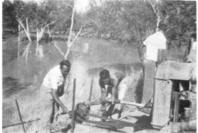
When the floods caused so much havoc at Brewarrina everyone got together in a great community effort. Here we see a temporary pump being installed.
